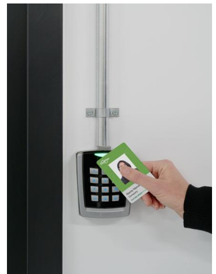
Intruder detection and cards throughout the data centre
